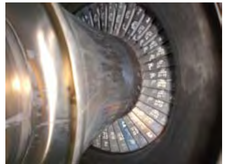
Power turbine and flange covering propeller gearbox
